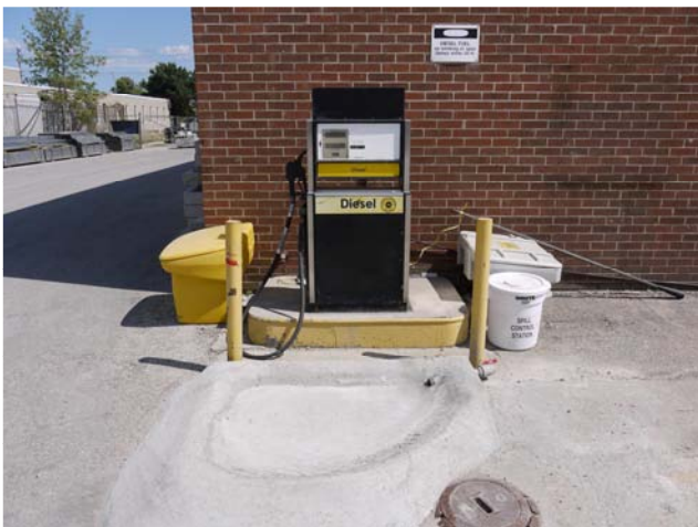
Spill containment sump installed
